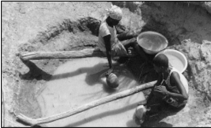
▲ Fig. 1. Fugu Alale and Awini Apam collecting water from the old source at Zeog-Bukin, Bolgatanga – site of well construction. Courtesy WaterAid/Caroline Penn.
